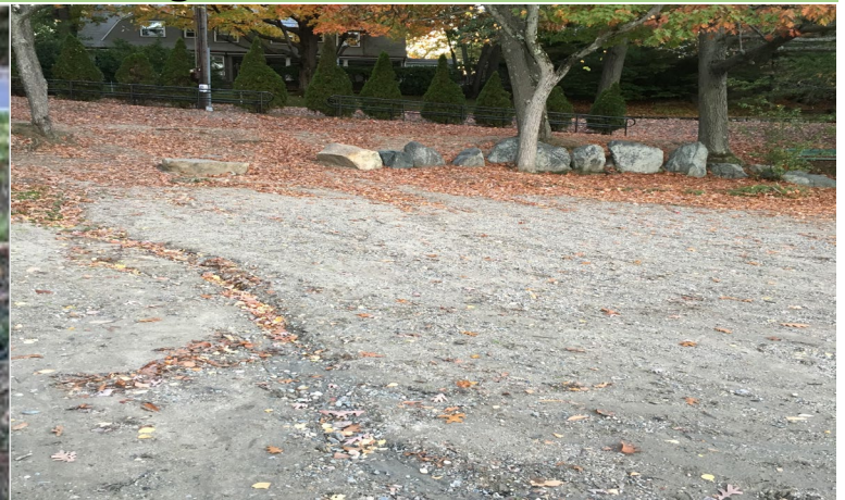
Levingston Cove eroded sloping lawn to the alcove
