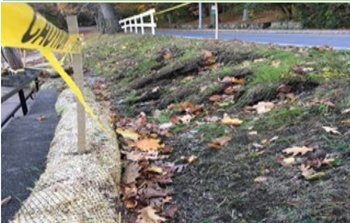
Levingston Cove fishing wall slope erosion
